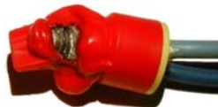
Loose wire connections create a high resistance point within the electrical system, which can lead to a breakdown in insulation or even a fire.
